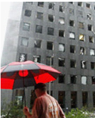
The first three floors of every building were completely uninhabitable after the storm.
